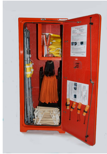
JB20EE with emergency equipment (supplied by others)
